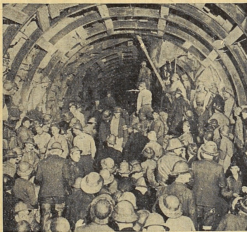
Completing a five-year job, hard-rock men holed through in the San Jacinto tunnel recently. Within a few months 1,000,000,000 gallons of the Colorado river will rush through this 13-mile bore daily in its haste to quench the thirst of Los Angeles and 12 other southern cities. It was one of the biggest tunneling jobs ever attempted.
