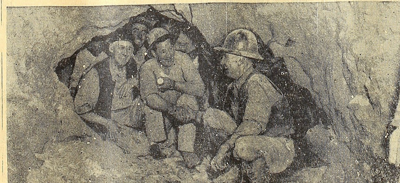
THAT'S HOW TUNNELS ARE BORN . . . The final "breaking through" of the rock barrier where the two sections of the Brooklyn-Manhattan tunnel join underneath the waters of New York harbor took place with a considerable bang as a dynamite charge was used to blast a hole through the last few feet of rock separating the two ends of the tunnel. The project, which has been under construction since 1940 and will cost 70 million dollars, is expected to be open for motor vehicle traffic in 1950. Above, Sam Allen, superintendent of the Brooklyn section, shakes hands with Andy Amisano of the Manhattan section.
