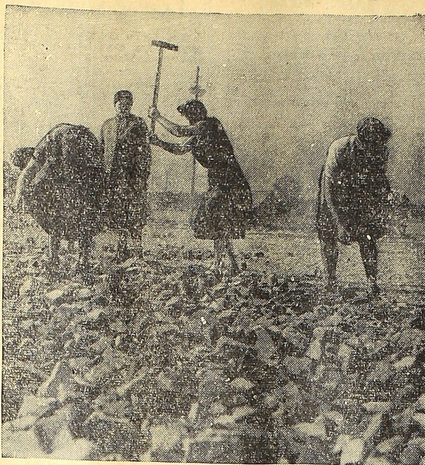
HELP ALLIED AIRLIFT . . . In order to increase the potency and efficiency of the Allied airtift into beleaguered Berlin, more air strips had to be built. Scores of German women, like those pictured above, are aiding the Allies by helping to build a new runway at Tegel, in the heart of the French sector of Berlin. These new strips relieve the heavy burden from the Tempelhof airport.
