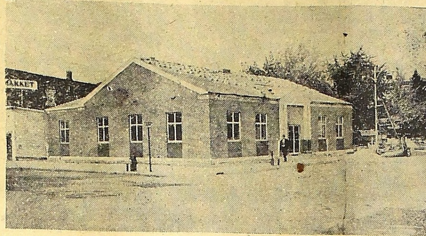
New Peoples State Bank Building of East Tawas is nearing completion. Workmen are now putting on the tile roofing and finishing the beautiful entrance to the building.
