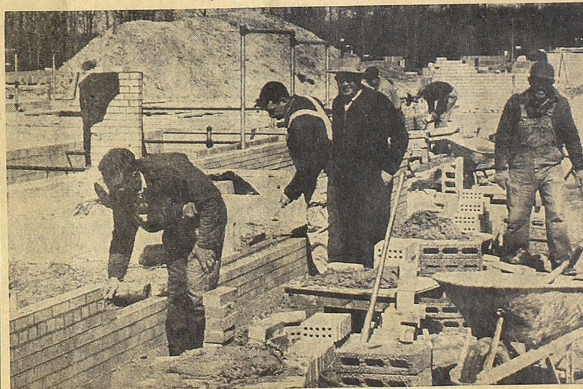
Jack Miller, Vollmer Construction Company superintendent, and crew laying brick at Tawas Memorial Hospital. The work is progressing according to schedule with completion date for construction early next fall.—HERALD PHOTO.
