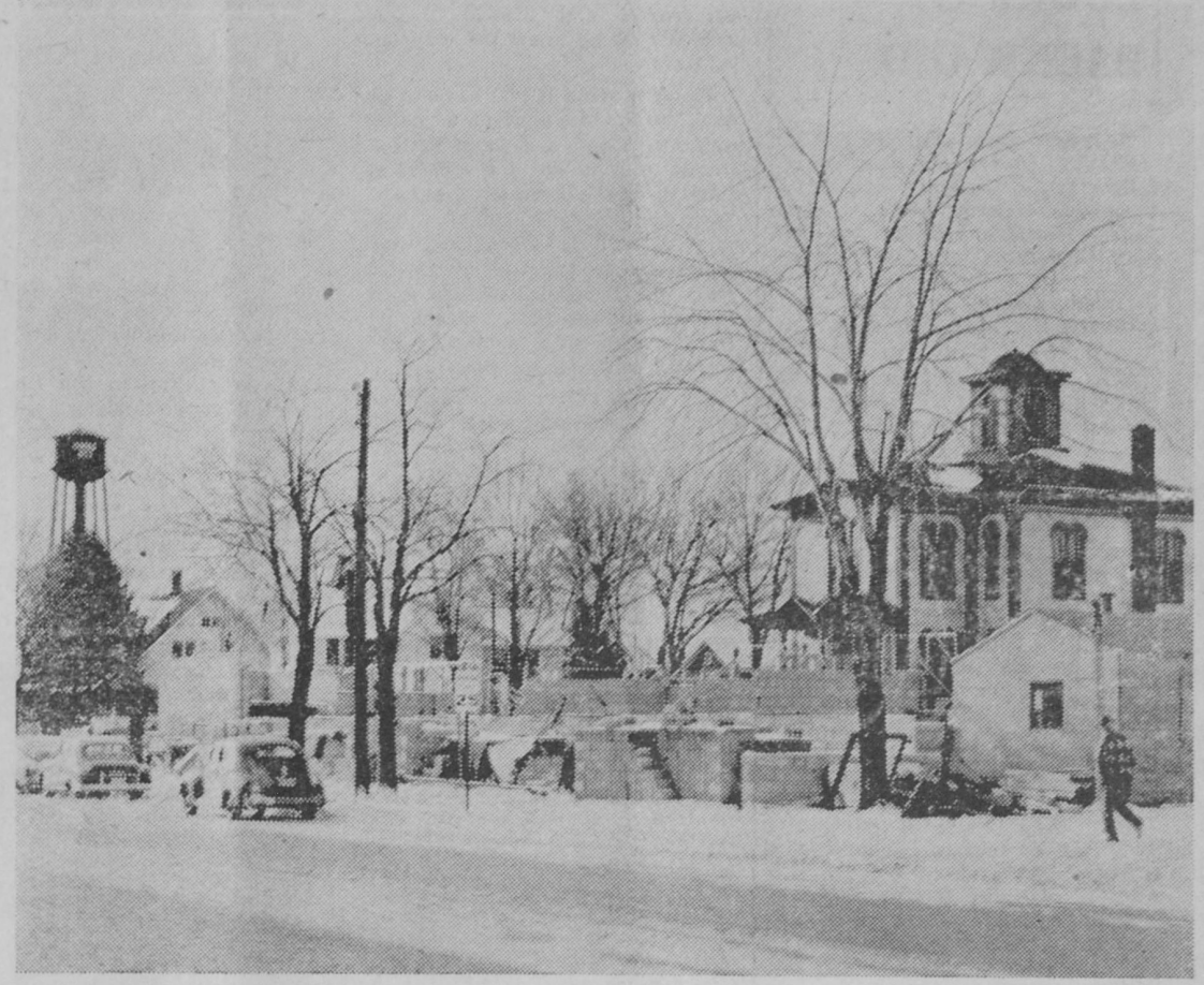
A large amount of work on the new Iosco County Building on Lake Street has been completed during last fall and early winter. Photo taken Monday.
