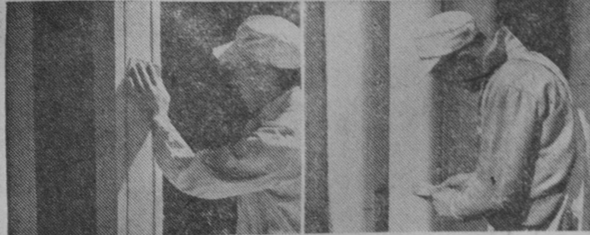
If the old paint is only slightly rough, sandpaper will do. A putty knife will effectively scrape away small areas.
