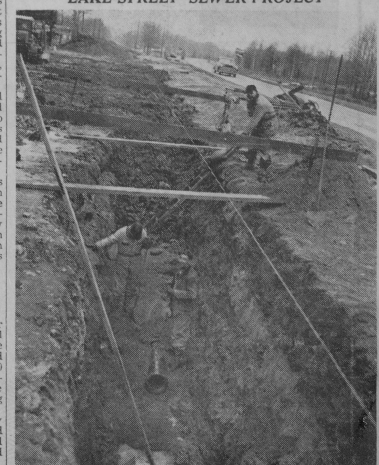
Rapid progress has been made during the past winter on Tawas City's Lake Street sewer project. Under the direction of Martin Kasicchke, superintendent of public works, a minimum of hand work has been used in its construction. When completed it will service the city's newest residential and business subdivision.—Herald Photo.
