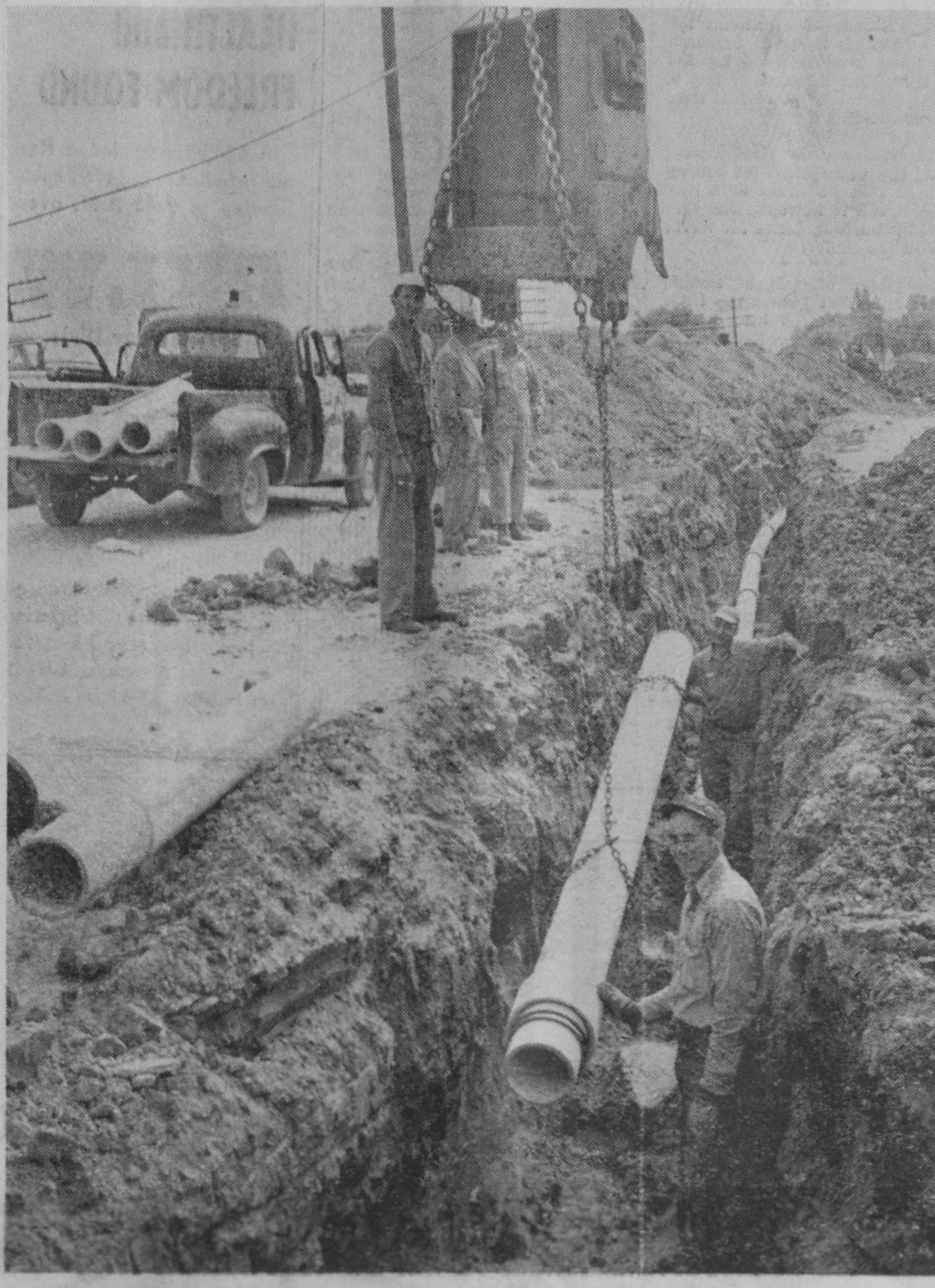
Dropping final section of force sewer main into place at the Lake Street pumping station last week Thursday which when completed gave this growing business and residential area of the city sanitary sewer service. Service started this week. The project which was under the supervision of Martin Kasichke, public works manager, and Clifford Spicer, city engineer, includes 3,380 feet of force main, 1,100 feet of sewer main and two pumping stations.—Herald Photo.
