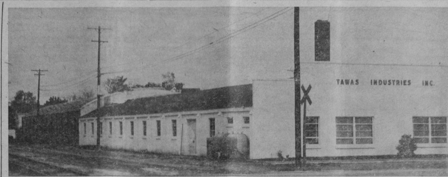
During the break in the weather this week, workmen were busy putting the roof on the new addition to the Tawas Industries plant in Tawas City. The new addition can be seen at the rear of the plant. The new 54 by 143 feet concrete block structure will provide warehouse facilities for the plant. The new addition will make the plant a full block in length, with an inside loading entrance on Wheeler Street and the main entrance on First Street. The masonry work is being done by James Boomer and the carpentry work by Edward Doak.—Herald Photo.
