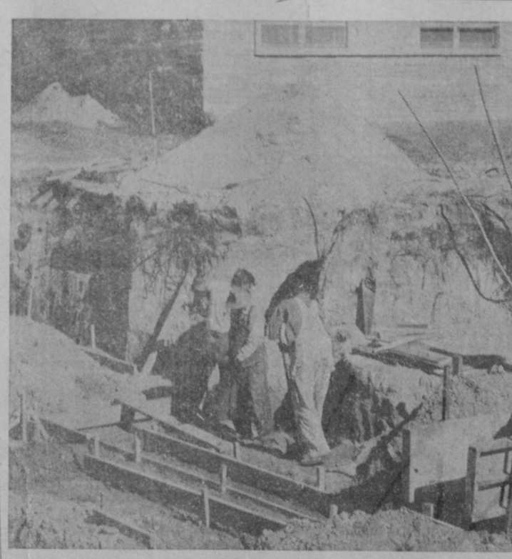
In the above photo, Davison-Rose workmen are shown constructing foundation forms for the new Isosco County Jail which is under construction. The contractors poured the initial concrete forms on Thursday of this week. Shown at the far right is Olaf Rose, a partner in the contracting firm. A portion of the new Isosco County Building can be seen in the background.—Herald Photo.
