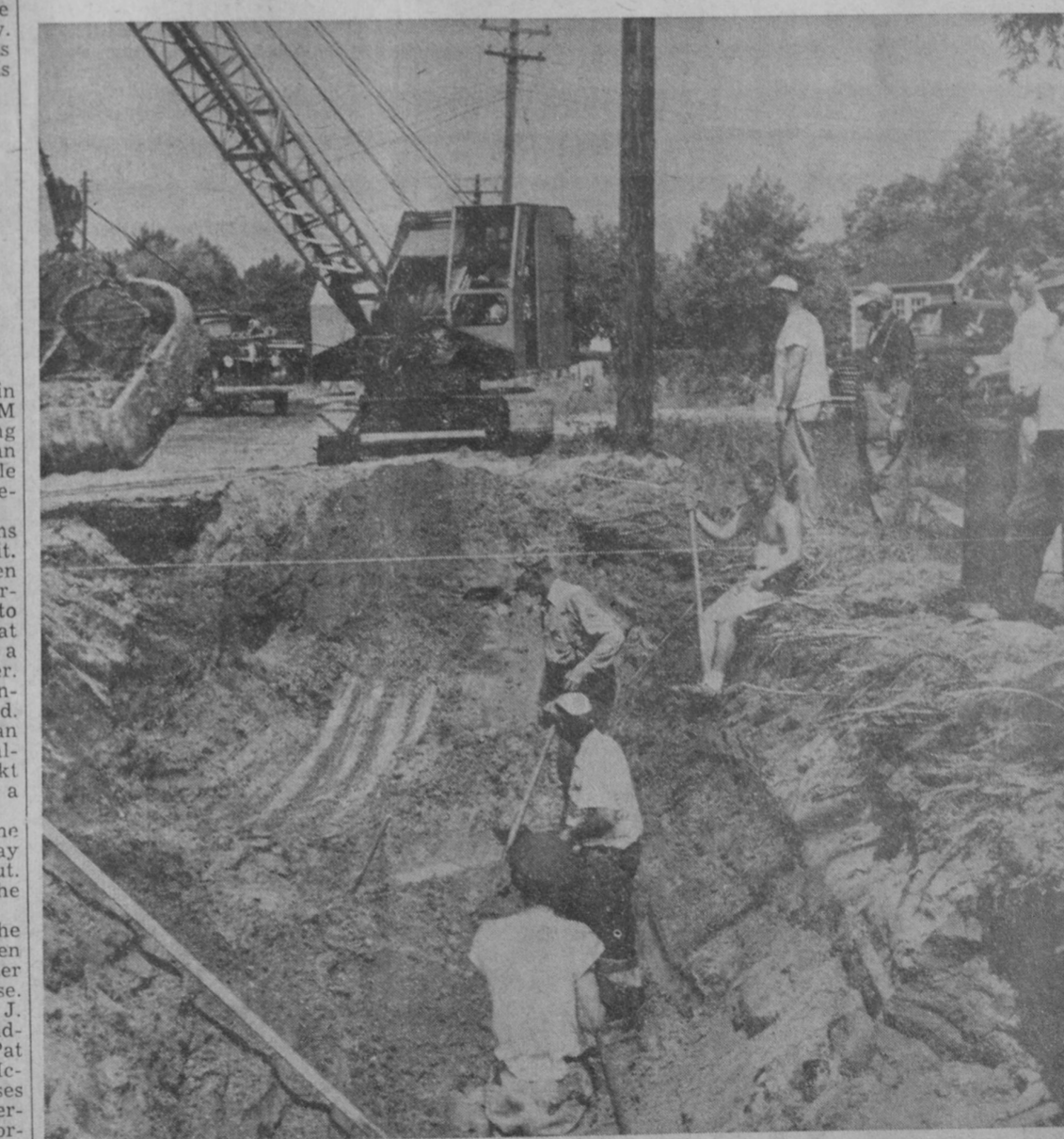
Work on the Harris Avenue sewer extension in Tawas City has progressed to the corner of First Street. Alternate layers of quick sand and clay along the route of the extension has resulted in a short delay. In the above photo a drag line operated by Frank Chartier is shown excavating at the site. Considerable hand shoveling by workmen was necessary at this point due to an uncharted water main. Supt. Reginald Bublitz and Matthew Pfeiffer are shown in the upper right hand corner of the picture.—Tawas Herald Photo.
