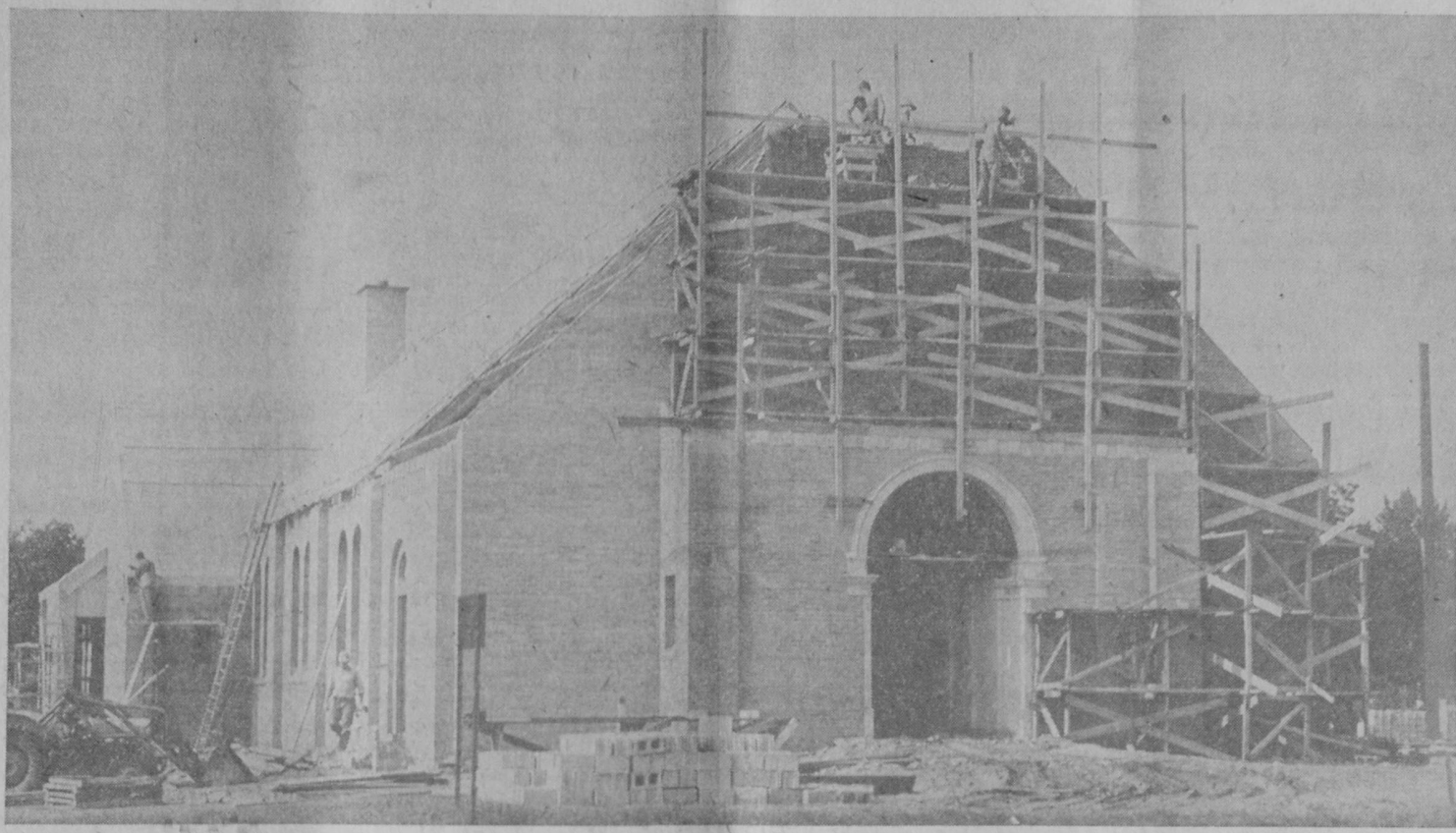
WORKMEN ARE SHOWN laying brick at the new Immaculate Heart of Mary Church in Tawas City. The picture, taken last Friday, shows the rapid progress on the front of the church. Cornerstone laying ceremonies will be held Sunday.—Tawas Herald Photo.
