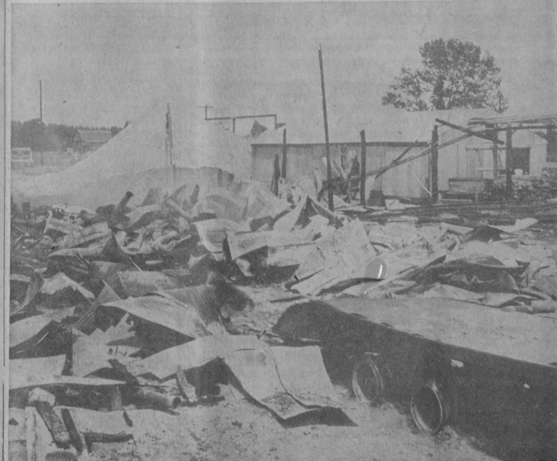
ONLY TWISTED METAL ROOFING and debris remains of the Bement sawmill on M-55 in Tawas City after fire consumed the main mill section last Friday morning. A huge pile of sawdust and one building is all that was left standing.—Tawas Herald Photo.
