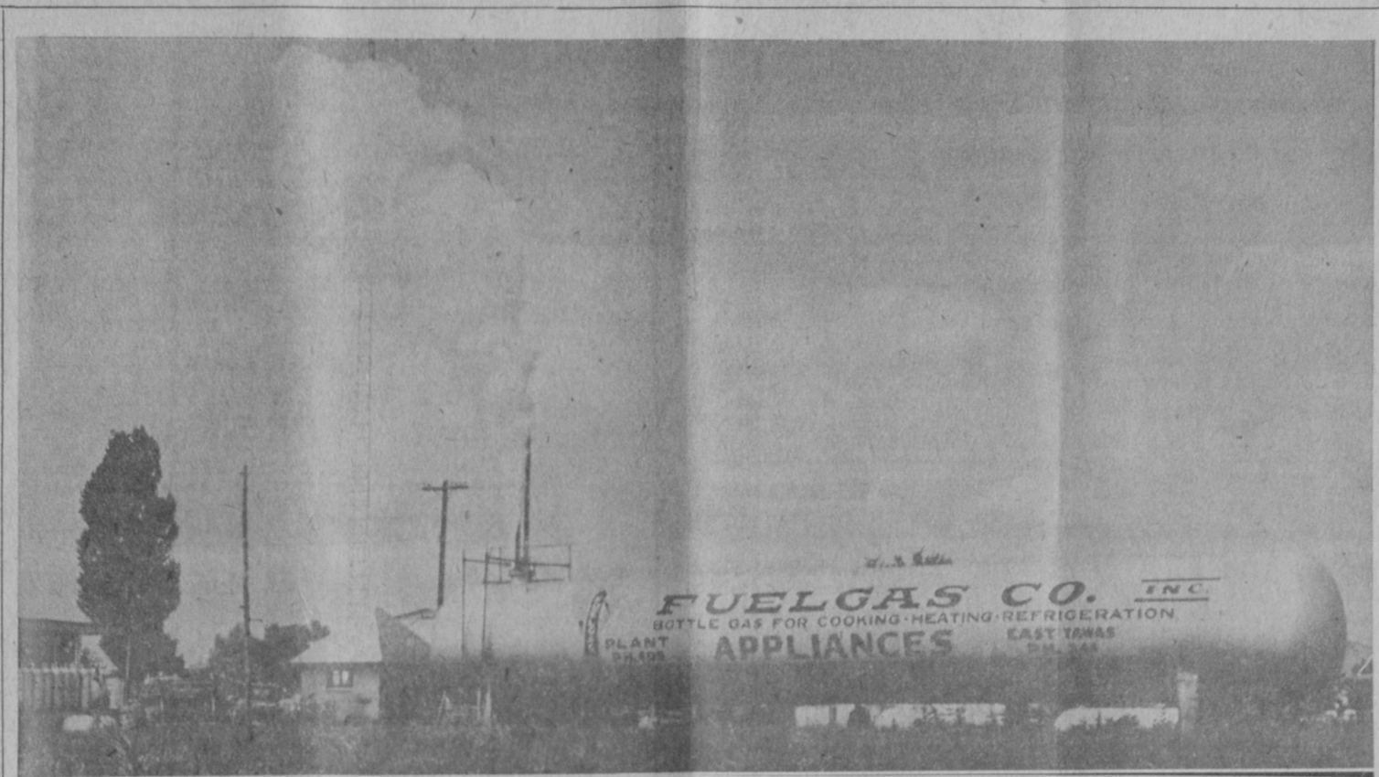
"BLOWING ITS STACK"—A white cloud of expanding liquid petroleum gas is shown spouting from a broken pipe in the center of the picture. Approximately 10,000 gallons of gas was released before the pipe was capped.—Tawas Herald Photo.
