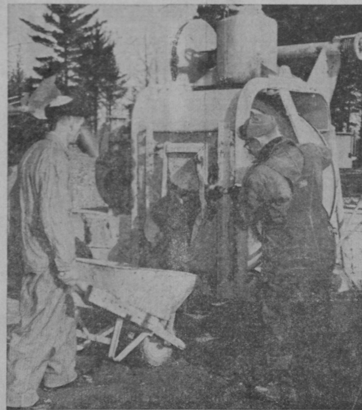
CONSTRUCTION IN THE TAWAS AREA was highlighted by the start of the new junior and senior high school.
