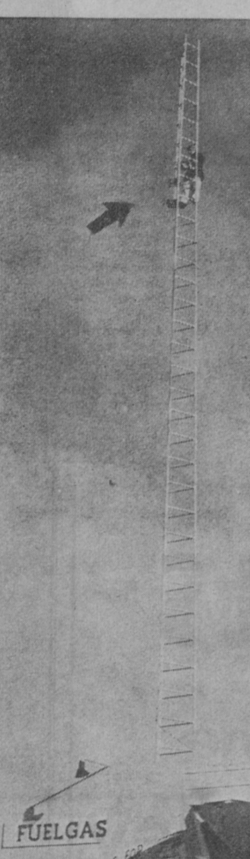
The arrow in the above picture points to a workman perched high on the 90-foot tower at the Fuelgas Company of the Tawas store in Tawas City. When the photo was snapped, the workman was preparing to install an antenna which is now being used on Fuelgas' new two-way radio system.
