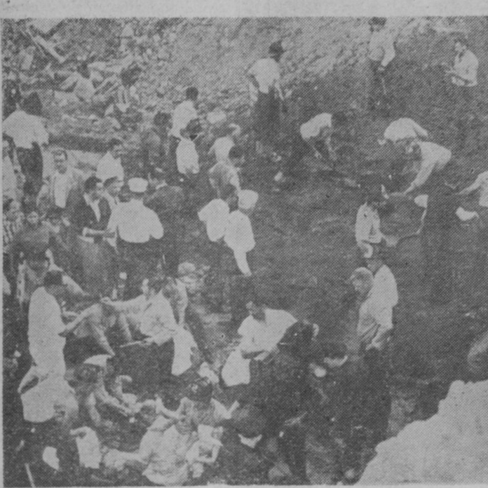
CAVE-IN TRAGEDY—This is the general view of the excavation site in New York where six children were killed when they were buried under tons of earth while playing in a 25-foot deep pit. Rescue workers can be seen working with pulmotors over one of the victims, a little girl. An investigation is now under way to determine responsibility for the apparently unguarded project.
