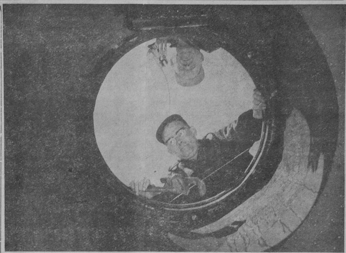
PEERING DOWN AN open manhole at the Bay Drive pumping station, in preparation for extension of sewer mains across US-23, is Reginald Bublitz, superintendent of public works, and Matthew Pfeiffer, foreman.—Tawas Herald Photo.
