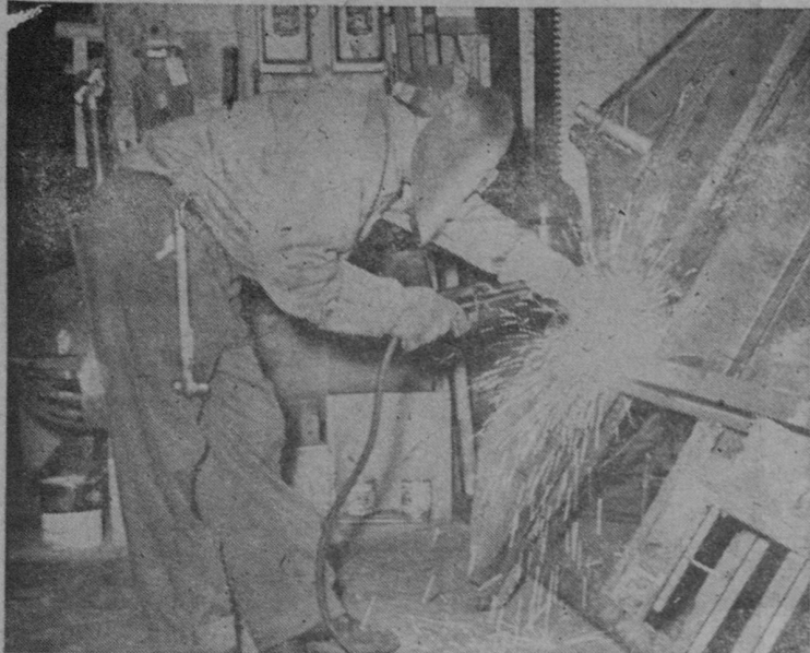
HOT SPARKS ARE FLYING as the frame for another Anderson is welded prior to being bolted to the wheel assembly as yet to be installed.—Tawas Herald Photos.
