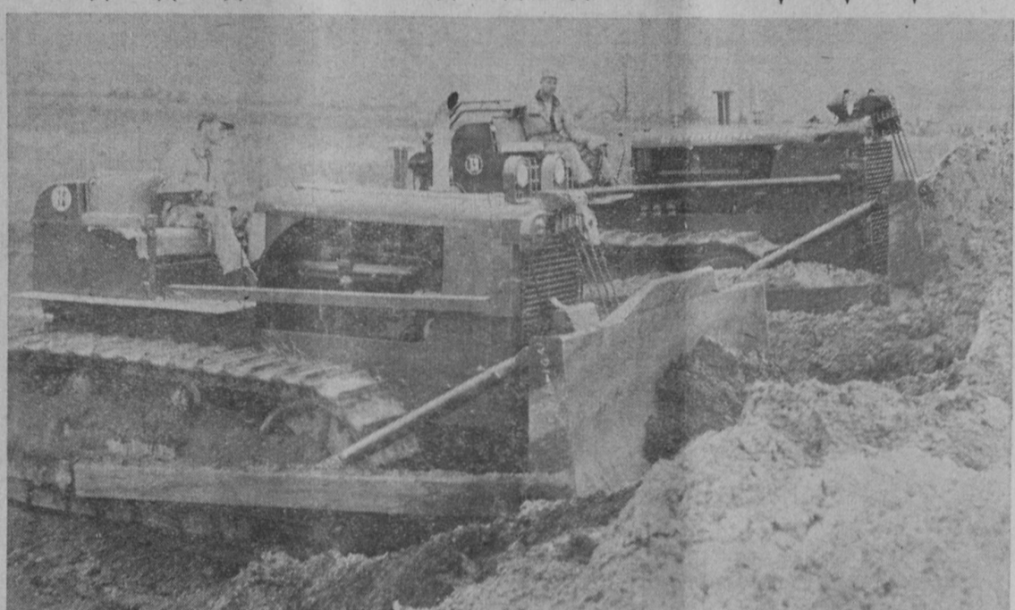
BREAKING GROUND FOR NATIONAL GYPSUM'S new quarry are these two bulldozers, operated by John Wallace of Hale and Donald Armstead of Whittemore. The process of stripping overburden from the deposit started last Thursday on the National City Road west of M-55.—Tawas Herald Photo.
