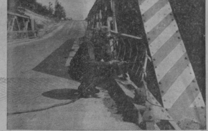
ENOS HAGLUND, road commission employee, cuts a smashed railing from the bridge after Monday's crash.—Tawas Herald Photo.
