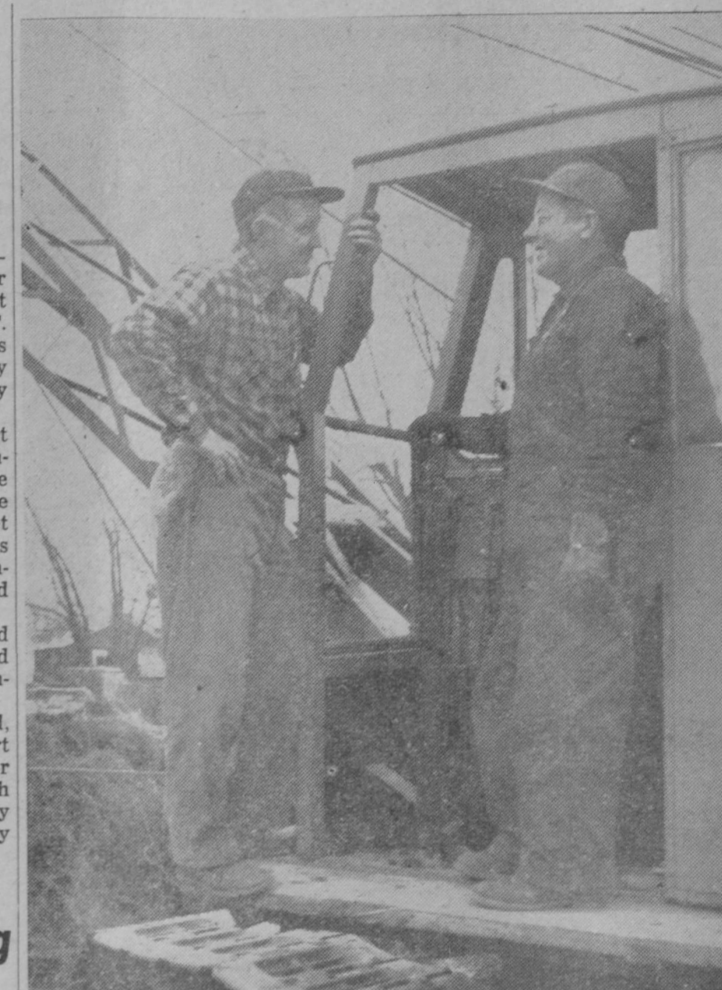
WORK STARTED THIS week on the small craft harbor at the Tawas River mouth. Myrl Kubic is at left, Frank Chartier, right.
