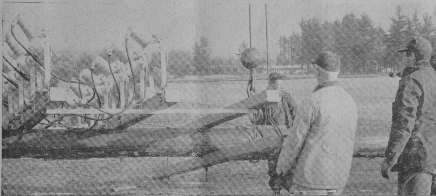
WORK ON SETTING the first pole at Tawas Area School's new athletic field is pictured above. John St. James of Tawas City, second from right, contractor for installing the lights, watches workmen prepare to lift the first 90-foot pole into place by means of a derrick. In the photo at right, a workman rides up to the top of the pole to free a fouled cable.—Tawas Herald Photos.
