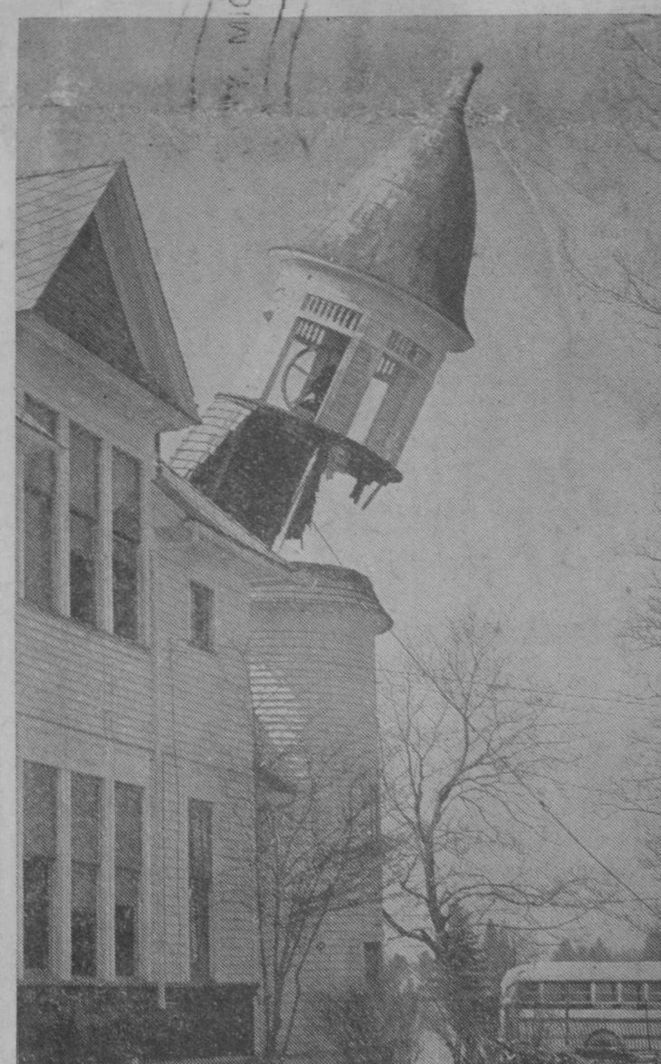
CAUGHT JUST BEFORE CRASHING to the ground is the belfry of the old Tawas City high school building. After sawing off timbers which supported the structure, a chain was attached and a truck yanked it to the ground. The tower buried its "nose" in the ground to a depth of about three feet. Workmen found under the galvanized steel roof the handiwork of carpenters of the 1890s. The curved portion of the structure was a lamination of one-inch boards, all planed and fitted by hand.—Tawas Herald Photo.
