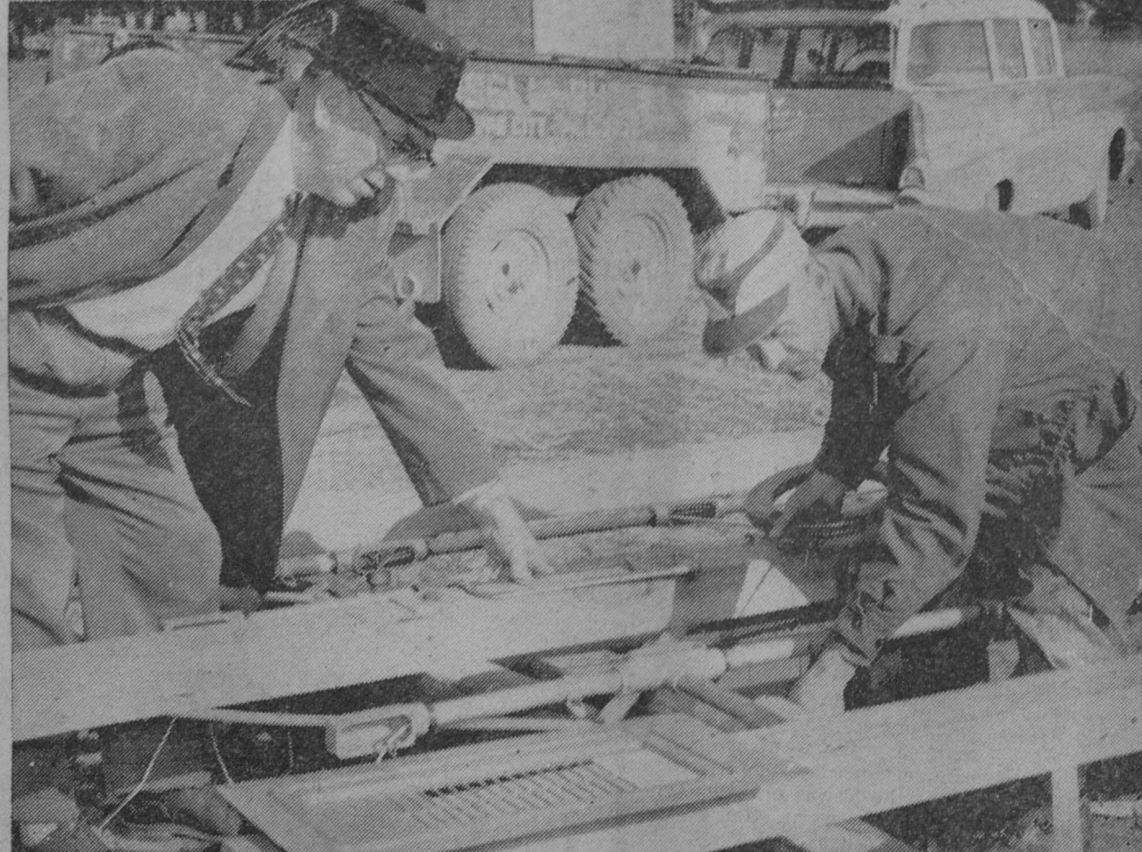
LIGHT POLES at Tawas Area School's new football field are expected to be set within the next two weeks if favorable weather continues. In the above photo, Supt. Reynold Mick is shown watching John Kindell of St. James Electric, Tawas City, contractors for lighting the field, as he installs electrical equipment on one of the poles.—Tawas Herald Photo.
