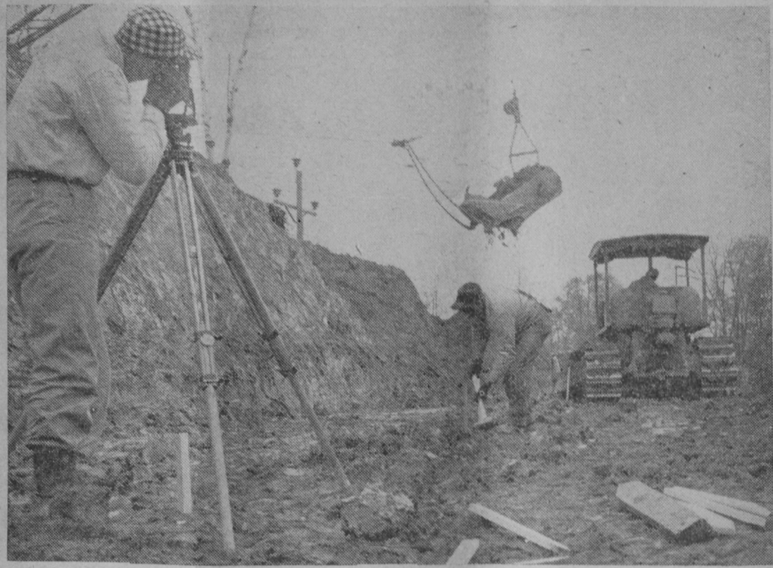
WORK IS UNDERWAY on crossing US-23 south of Tawas City for National Gypsum Company's conveyor system to transport rock to its proposed lake-loading site. In the above photo, engineers are shown "shooting a grade" with a transit. A bridge is to be constructed on US-23 similar to the one at Alabaster. General contractor is Atkins Construction Company, Detroit. John Konenske of Tawas City is subcontractor.—Tawas Herald Photo.
