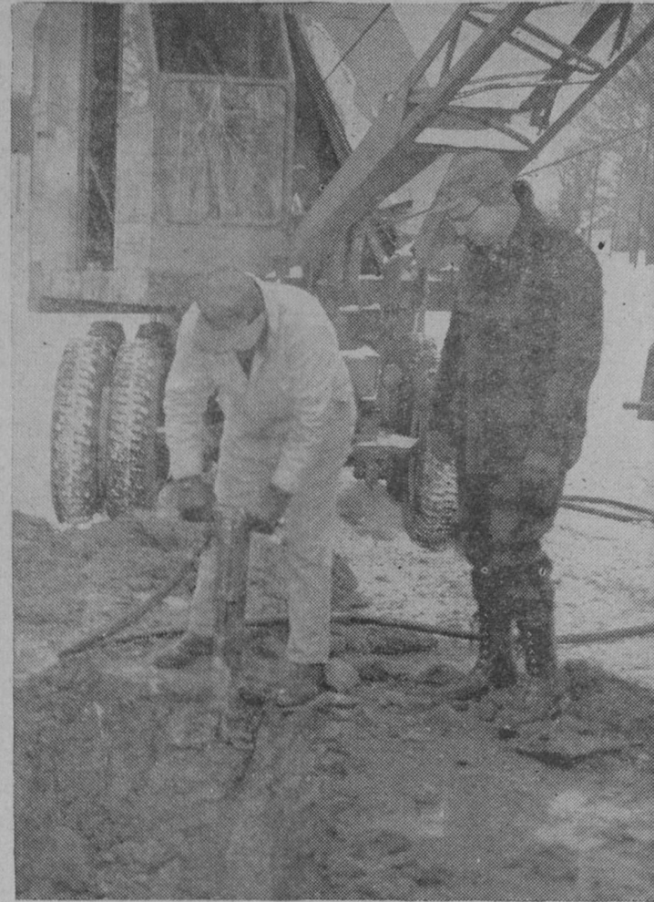
COLD JOB —The December cold wave caused a break in a four-inch water main on Whittemore Street Saturday. Supt. Reginald Bublitz watches Harry Gaul as he breaks up the frozen ground with an air hammer in preparation for repairs.—Herald Photo.
