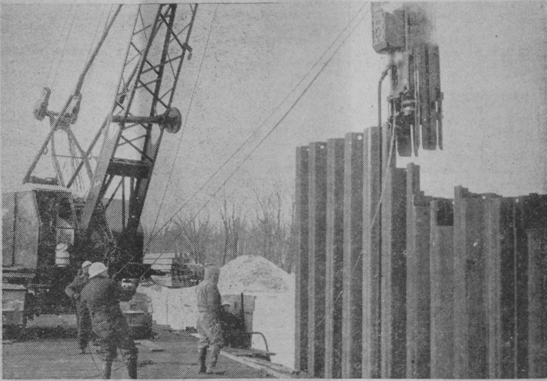
WORK ON steel caissons to support an overhead tramway system at National Gypsum Company's lake loading site south of Tawas City is pictured here. Construction has continued through the winter months. A steam pile driver is in operation here.—Tawas Herald Photo.
