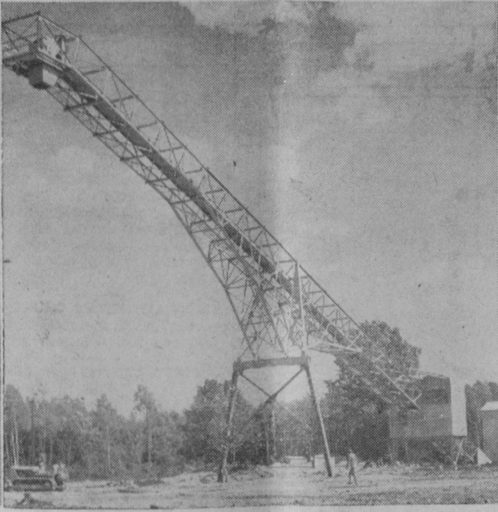
MUCH WORK has already been completed at the shore loading site. Pictured here is a huge conveyor which transports raw gypsum rock to the underground conveyor belt leading to shore.
