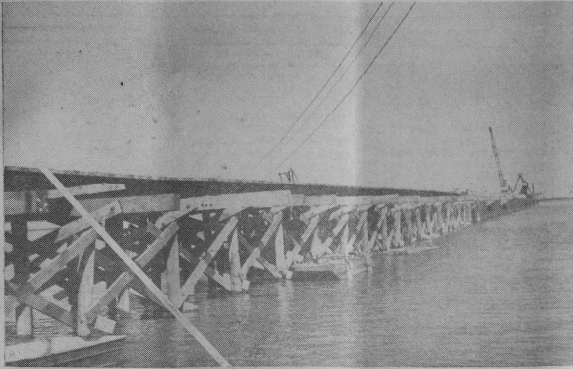
THIS IS THE temporary pier which National Gypsum Company has constructed south of Tawas City in Saginaw Bay to facilitate construction of its new aerial tramway. A dragline is pictured at the far end working on the last caisson crib for the structure.—Tawas Herald Photos.
