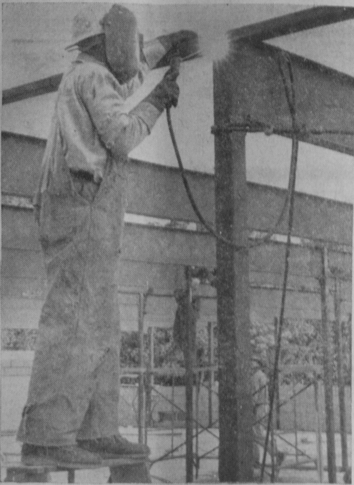
A WELDER is pictured above working on steel work at the new Whittemore-Prescott Area School which is now under construction. Turn to page 5 for another picture.—Tawas Herald Photo.
