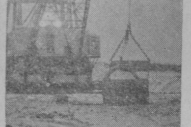
AT DUSK—This huge Marion dragline is shown operating by means of floodlights. Turn to page 10 for more pictures.
