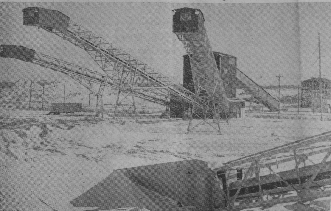
HUGE ARMS containing conveyor belts extend out from the screen house in the center of the picture. The rock first goes through the crusher building, at right, through the screening operation and then to stock piles. A conveyor belt in the foreground moves the rock underground to the car loader.
