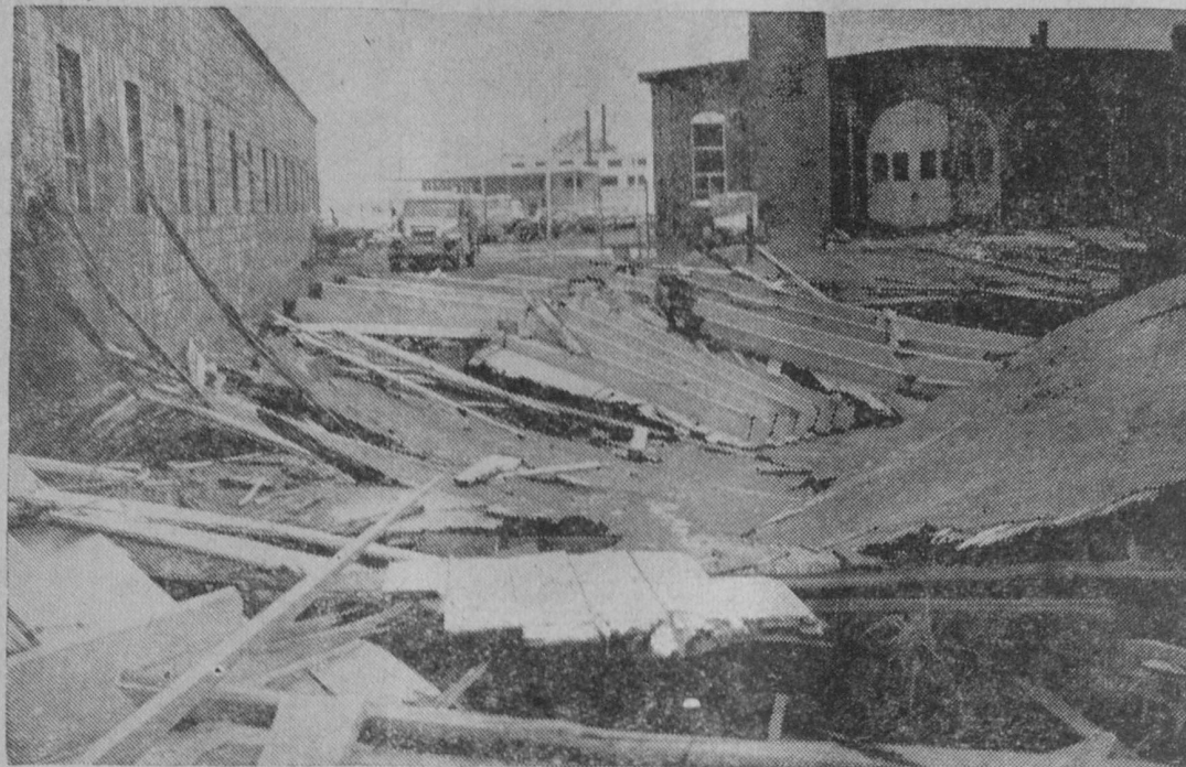
HERE IS THE ROOF of Feather-Lite Company's building after it was torn off in Sunday's storm. The wind "picked" the roof up and then smashed it into the ground behind the building.—Tawas Herald Photo.
