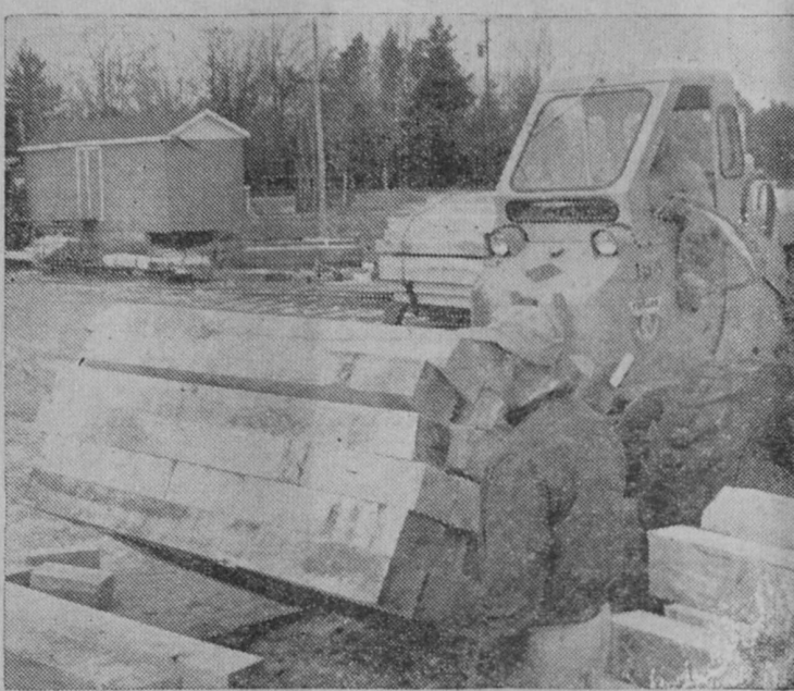
A LIFT TRUCK is used to transfer stacks of guardrail posts to the retort for Osmosal treatment.—Tawas Herald Photo.
