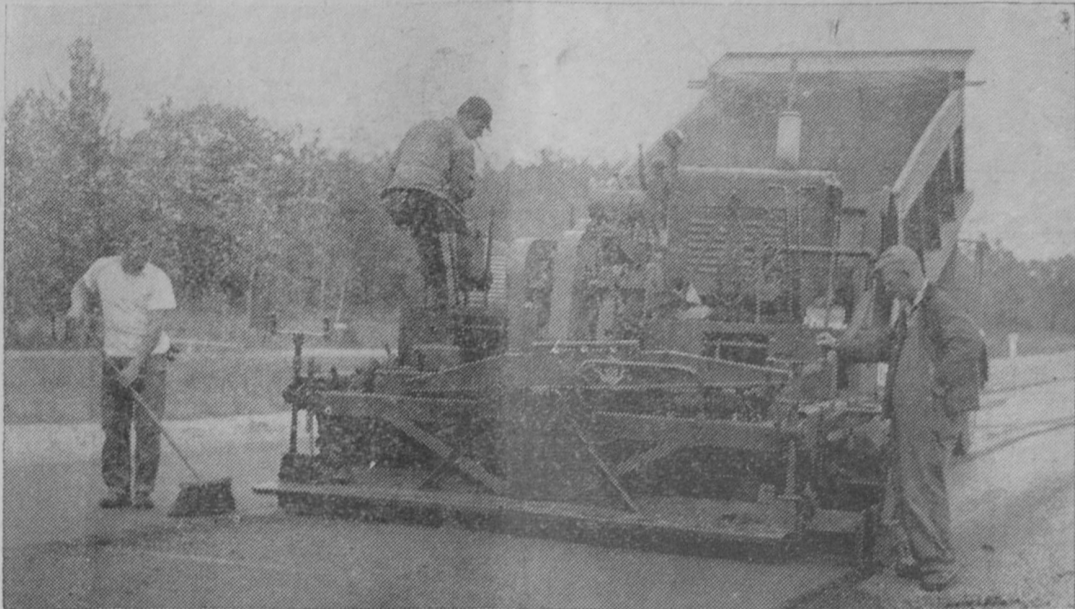
THIS WAS THE SCENE last week as Williams Brothers Asphalt Paving Company of Ionia was speeding work on surfacing M-55 east of the M-65 intersection. The firm has until the first week in November to complete this stretch of paving. State highway department regulations do not permit construction after that time. Work is progressing rapidly and the contractor believes the job will be completed by that time.—Tawas Herald Photo.
