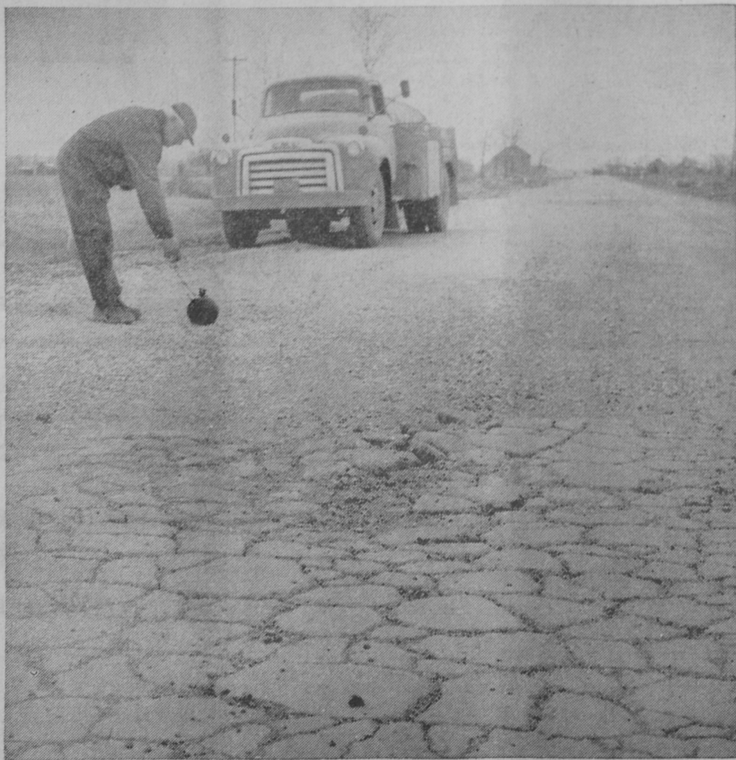
The "PRIDE" of Eastern Iosco County during the 1950s, heavily traveled M-55 from Hemlock Road Baptist Church east to Tawas City, is again a motorist's nightmare. The past winter and recent spring thaw saw this less than 10-year-old stretch of asphalt pavement break up in many sections. The picture above was taken east of the church and shows Allen Brown of the Iosco County Road Commission setting out a flare to mark one of the worst sections. Loose pieces of asphalt, shown in the foreground, are ready to "pop" out of place because of traffic. A considerable amount of patchwork has been done on the road with more to come.—Tawas Herald Photo.
