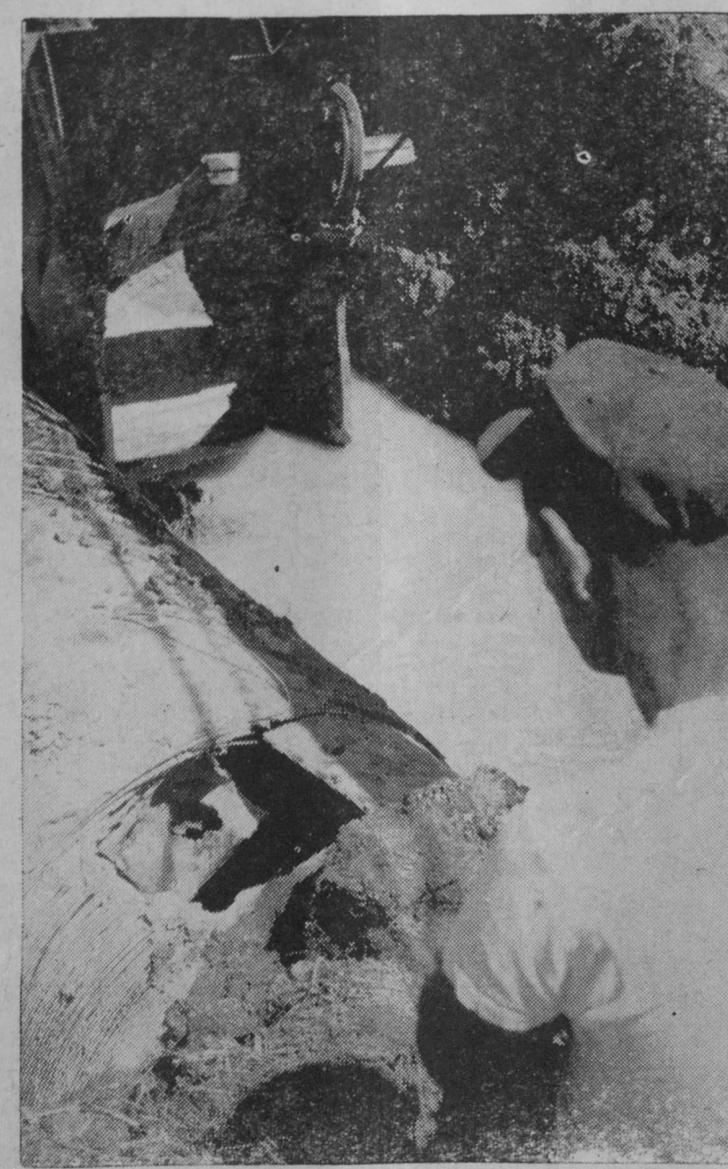
A BREAK in a 48-inch water main between Whitestone Point and AuGres Saturday disrupted service to customers of the Saginaw-Midland Water System. A workman is shown in the foreground looking at the hole in the top of the pipe.—Tawas Herald Photo.
