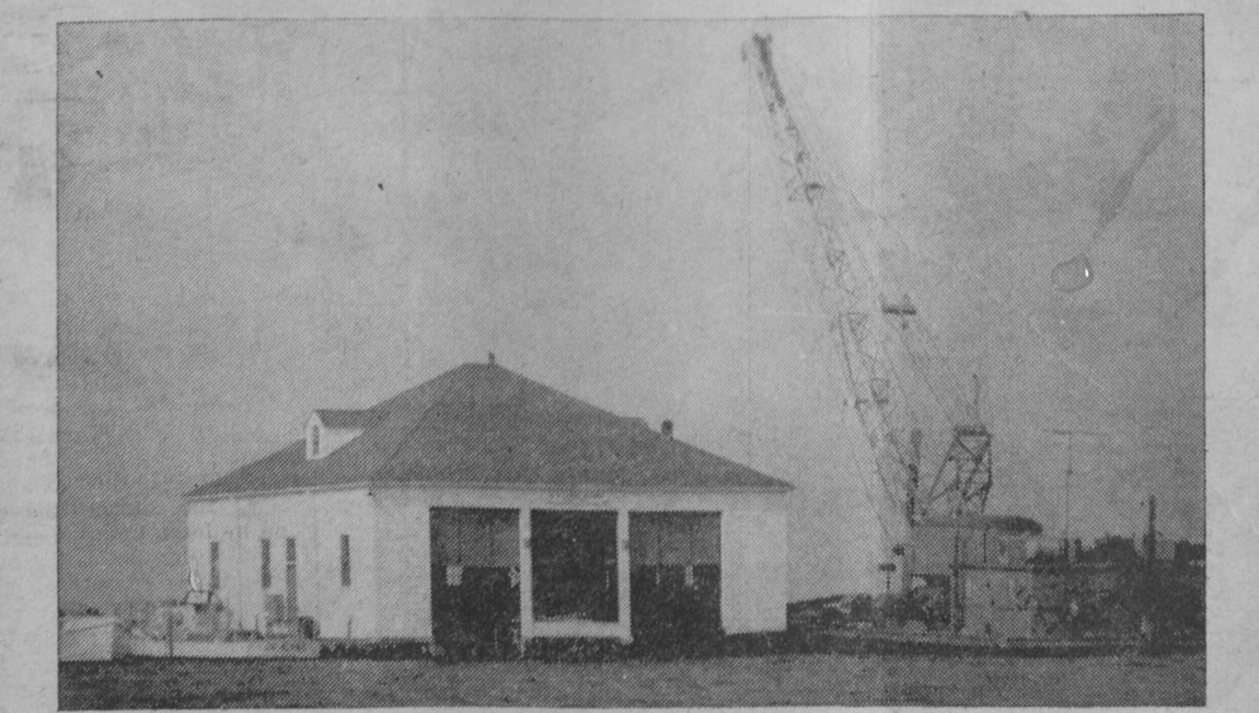
MORE THAN $20,000 in repair work is being done on the United States Coast Guard's boat-house at Tawas Point. Old piling and cribbing which has deteriorated through the years is being replaced. A coast guard barge from Toledo and crew of five men is shown in the above photo
