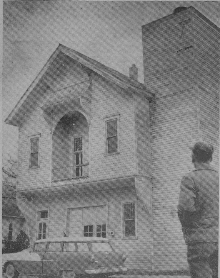
WORK STARTED MONDAY on razing the old city hall at East Tawas as plans were announced to construct a new building.
