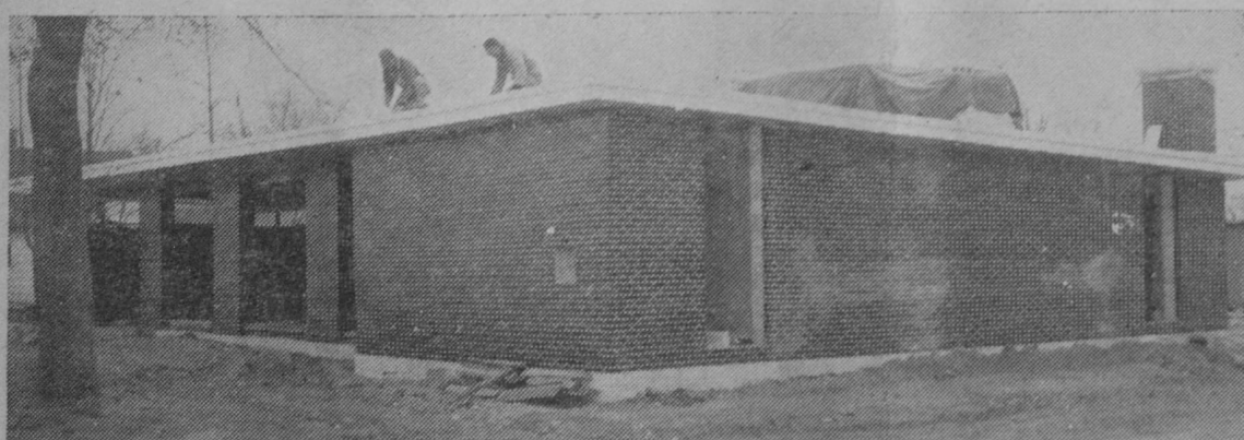
PROGRESS on the new Tawas City branch of Peoples State Bank is shown in the above picture, which was snapped Tuesday morning. The building is of concrete block construction with a facing of glazed ebony brick. Steel roof decking on the structure was installed last week. The new building is located on US-23.—Tawas Herald Photo.
