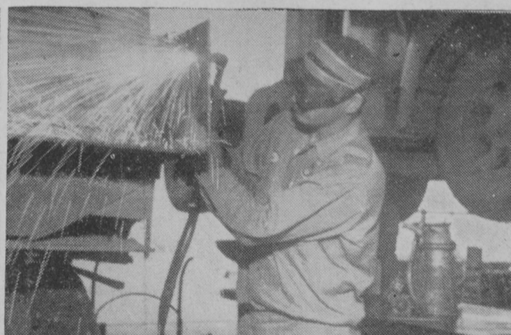
Hot sparks are flying as Dale Barber, mechanic and expert welder, installs a spreader apron on a husky RF-192 International tandem dump truck.
