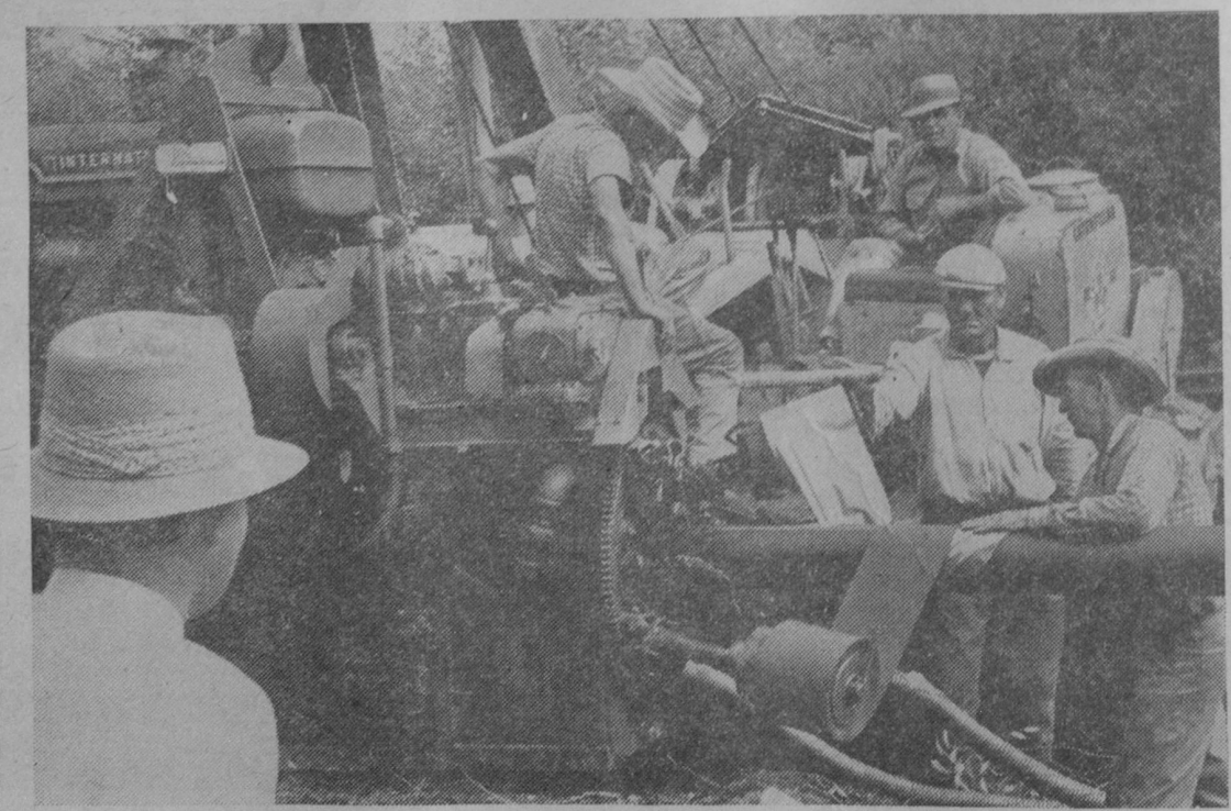
WORKMEN are shown applying "mummy wrap" to the pipeline above. Watching progress at left is Stuart White, traffic manager for the Detroit and Mackinac Railway Company.—Herald Photo.
