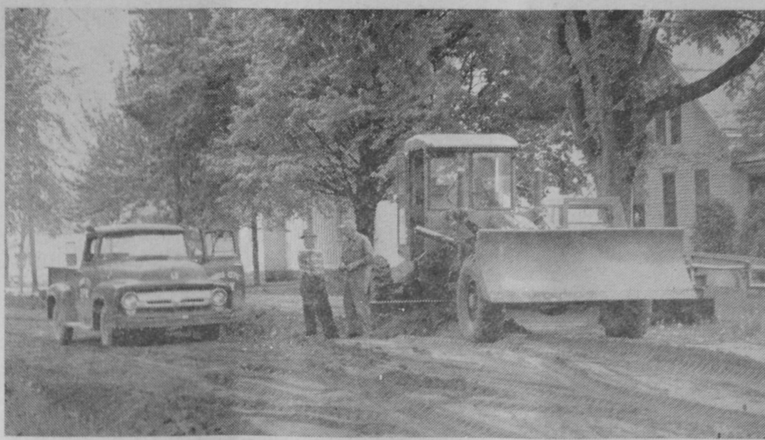
TAWAS CITY'S spring street construction program started last week. A. J. Merrill, local heavy equipment operator, started work on about 400 feet of Fourth Avenue from Mathews Street to Whittemore Street. The roadbed is being readied for seal-coating, which will take place the last week in June. Merrill is shown here with City Foreman Matthew Pfeiffer as they discuss the work.—Tawas Herald Photo.
