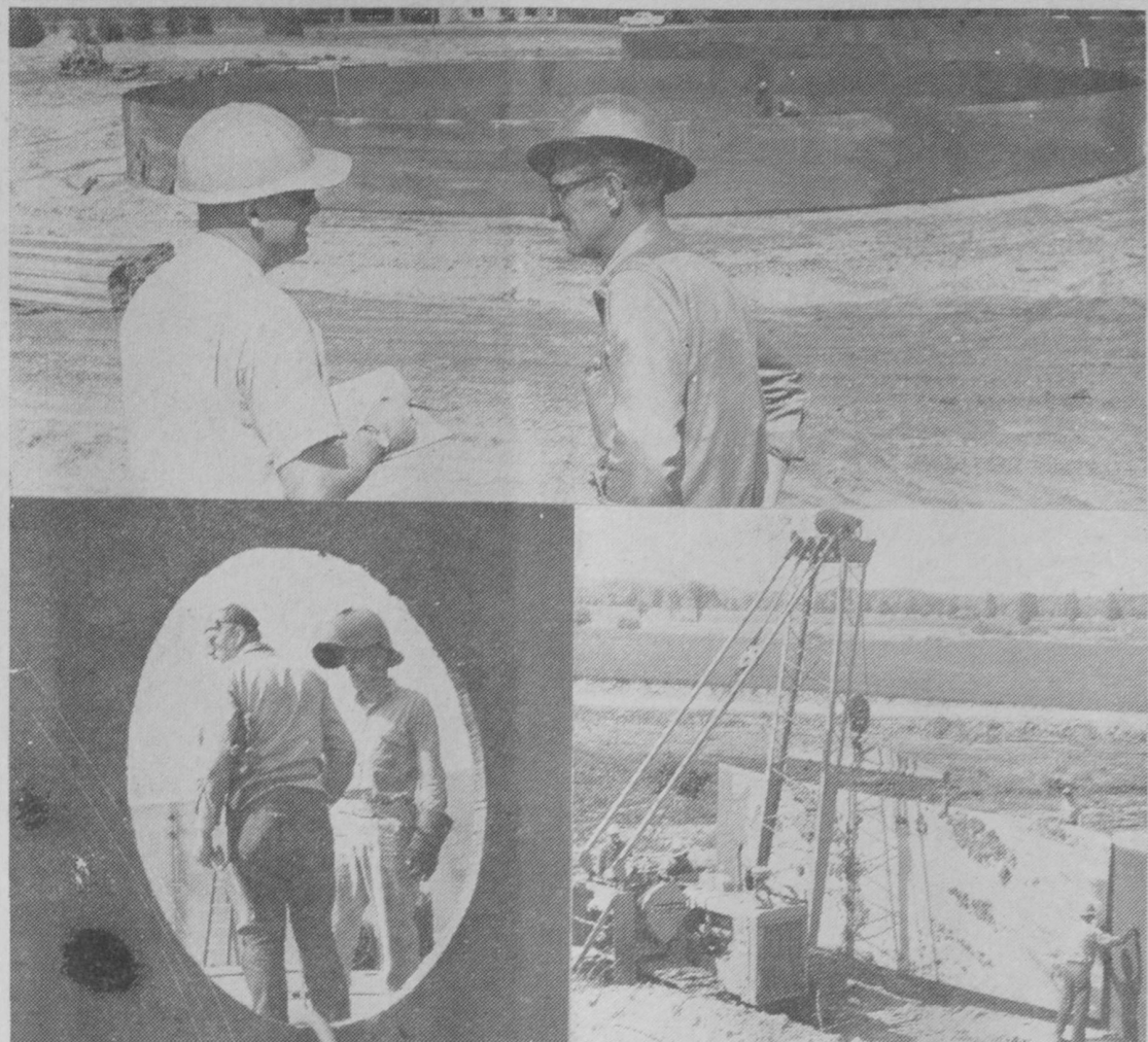
WORK IS PROGRESSING RAPIDLY on the 400,000-barrel terminal of American Fuel Oil Company at Harrisville. When completed, this huge installation will serve Wurtsmith Air Force Base at Oscoda. The company has received permission from the Michigan Department of Conservation to construct unloading facilities in Lake Huron for lake carrier transportation. A pipeline will move fuel from the ships to the terminal. The top picture shows Clifford Curry, left, resident engineer for Dwyer and Kite Construction Engineers, Kansas City, Missouri, and E. H. Force, right, superintendent for General American Transportation Corporation, Chicago, Illinois, contractor for constructing the tanks. Five huge storage tanks are being constructed north of Harrisville on US-23. Each tank, pictured at top in the background, holds 80,000 barrels of fuel. About 30 men are working on the tanks, which are being constructed of three-quarter inch plate. The tanks will have a floating roof. The pictures below show two welders framed in a tank aperture at left and at right a section of plate is being installed on a tank. The terminal is expected to be ready by September 1. —Tawas Herald Photos.
