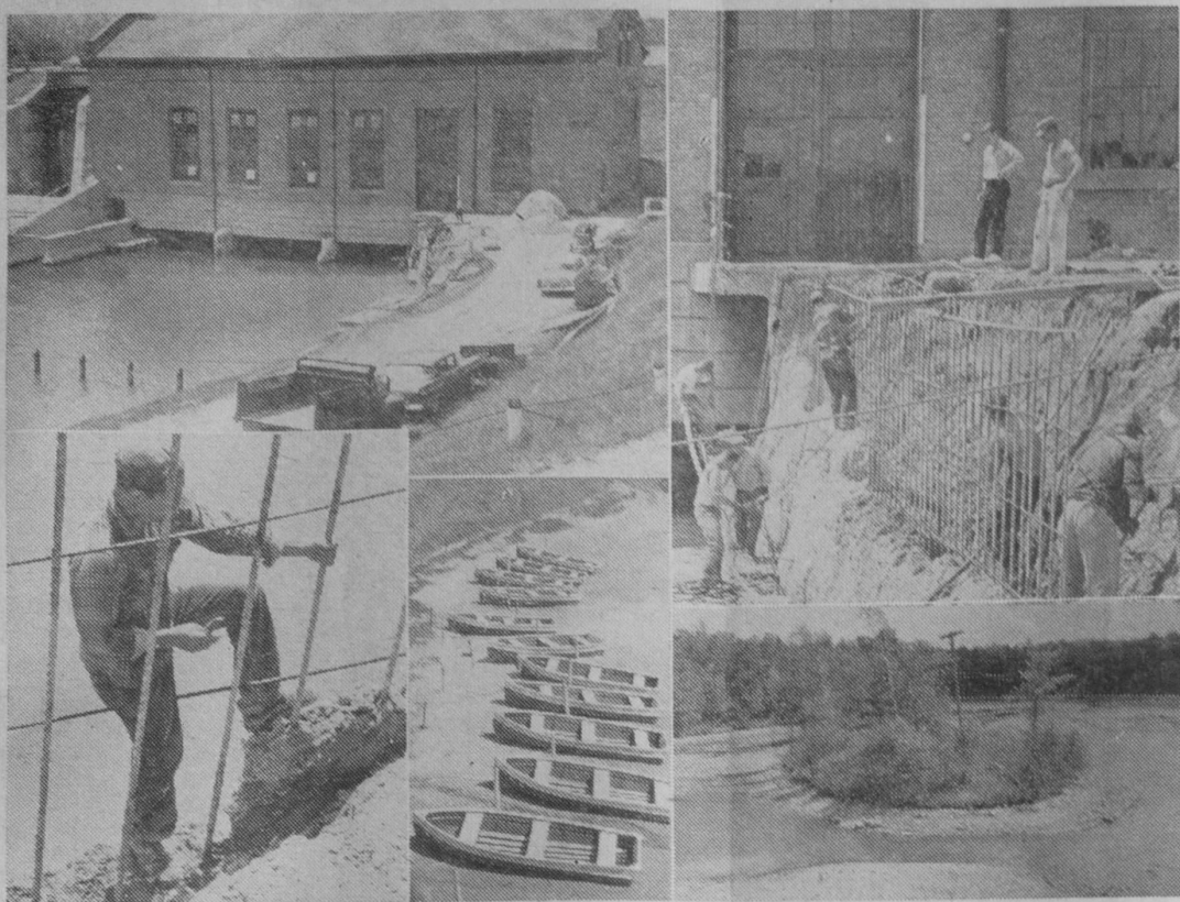
RECONSTRUCTION WORK on Five Channels Dam is shown in these pictures. At top left is an over-all view of the dam. At right, workmen are shown building a framework of reinforcing steel around one of the concrete retaining walls below the dam. At bottom left, a workman fastens the reinforcing steel in place while perched on a ledge over the river. The small inset in center shows the result of lowering the river pond between Cooke Dam and Five Channels. These rental boats have been left high and dry as the water was lowered four feet. The picture at bottom right was snapped from the M-65 bridge. Normally, the AuSable flows on both sides of this island, but due to the low water, the channel now flows on one side.—Tawas Herald Photos.
