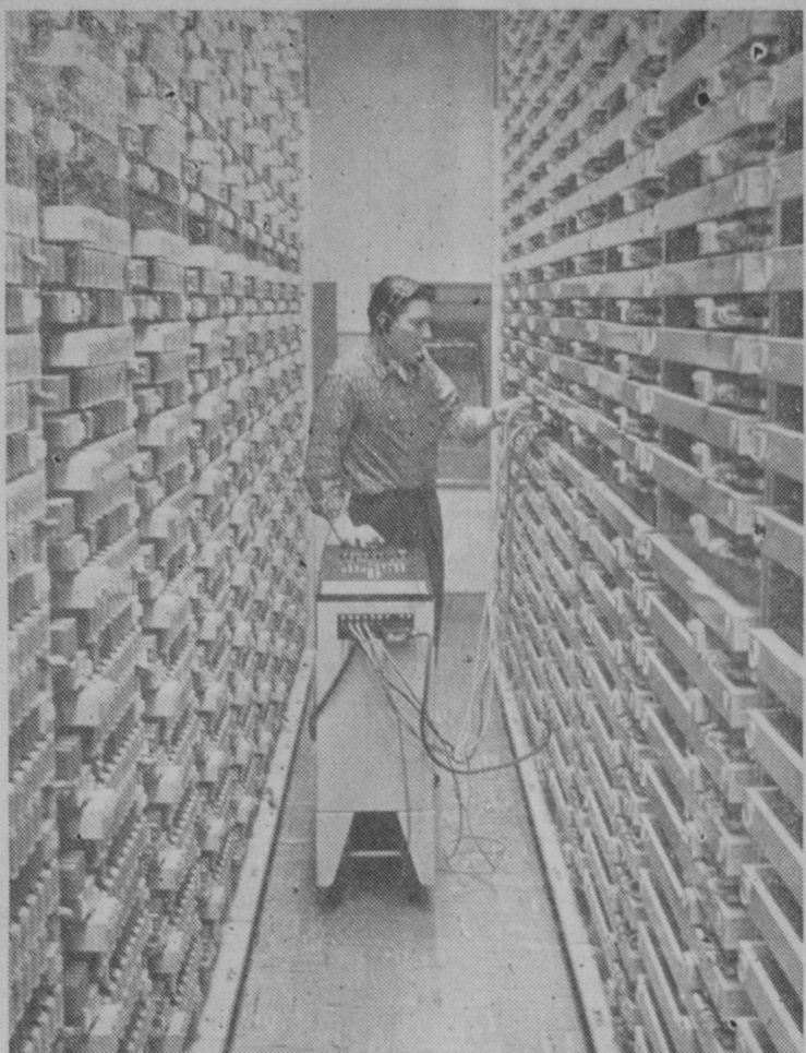
TRUNK TESTING —Frank W. Muessig, Michigan Bell switchman, tests out some of the lines that tie in with the nation's direct distance dialing system. This is part of the equipment which will put any one of about 45 million telephones in the United States and Canada within fingertip reach of telephone users here June 4, when the new long distance service is inaugurated.
