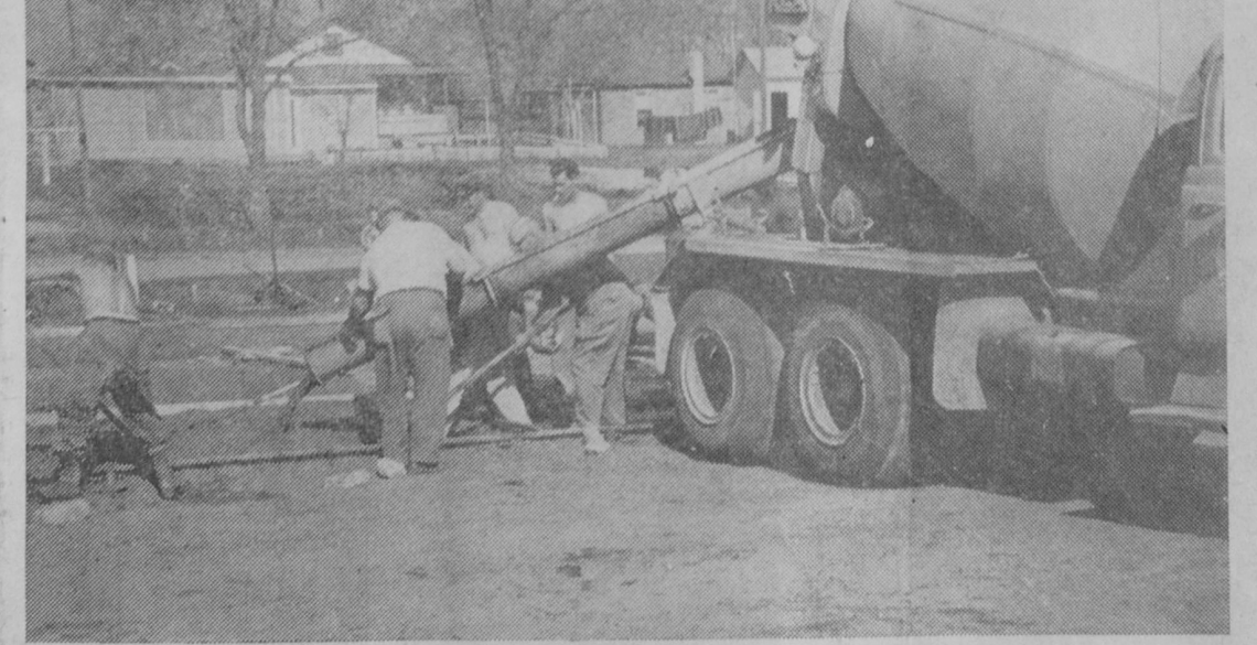
OSCODA HAS A new tennis court, brought about through the cooperative efforts of a large number of citizens who volunteered time last Saturday to work on the project. A crew of 20 persons turned out at 6:30 a. m. to perform the work of pouring and finishing the concrete slab, pictured above. Another crew had made preparations the previous day by setting forms. The new court was built over an
