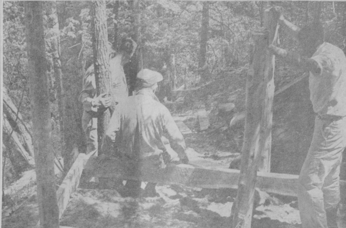
IT'S A LONG WAY DOWN—Volunteer workers who started reconstruction of the stairway leading to Largo Springs Sunday take a breather for a few minutes, as shown in this picture. The project is being sponsored by the Oscoda Park Commission and work will continue during the week. Another work bee is scheduled Sunday and anyone interested in furthering this attraction is requested to be on hand.—Tawas Herald Photo.
