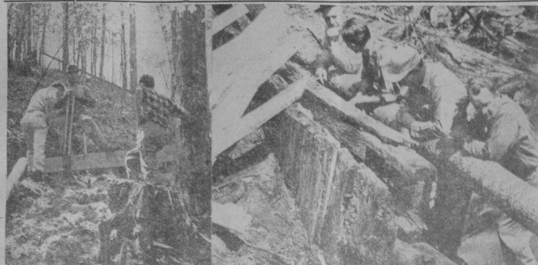
IT IS TOUGH TO CLIMB to the top of the slope at Largo Springs without the benefit of steps, pictured at left. These workers are building a new stairway. Howard Brubaker and his crew
