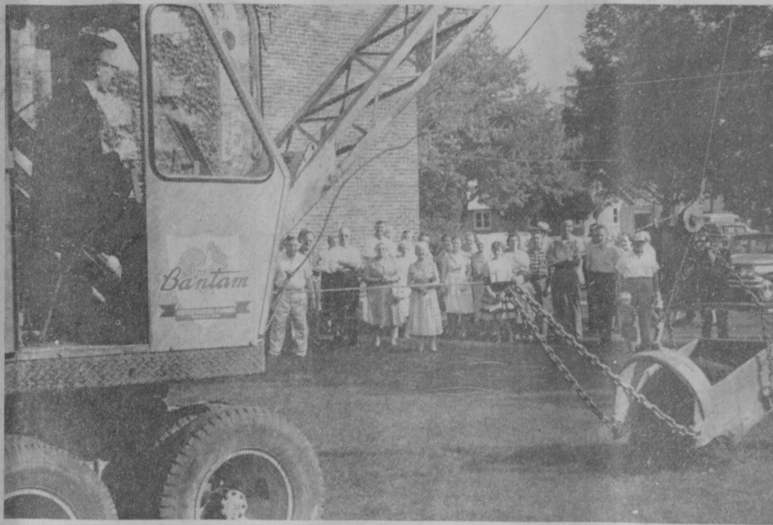
BREAKING with traditional ceremonies Sunday, Pastor Walter C. Pieper is shown at the controls of this dragline as sod was broken for the new Christian day school of Zion Lutheran Church. Members of the congregation watch the unique ceremony in the background.—Herald Photo.
