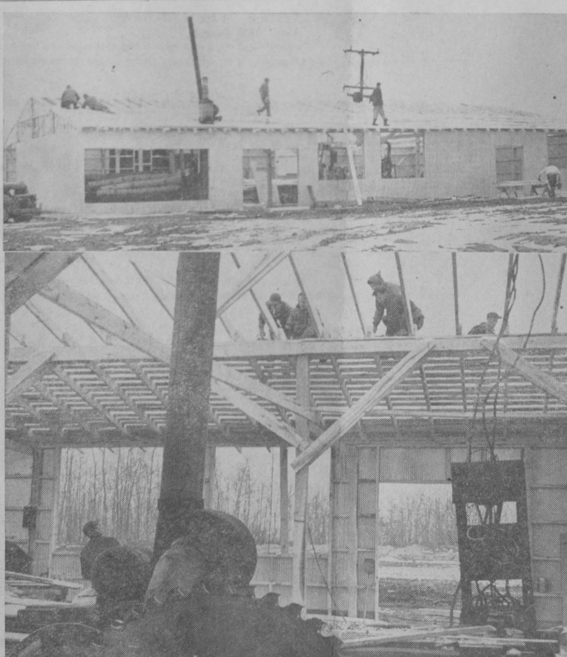
WORK IS BEING COMPLETED this week on the new frame and steel building which will house Hale Wood Products. The building is being constructed on the site of its former location which was destroyed by fire April 1. Exterior of the new structure is pictured at top as workmen were constructing the roof last Saturday. The bottom picture shows the interior. A large circular saw, which was saved from the flames, is in the foreground.—Tawas Herald Photos.
