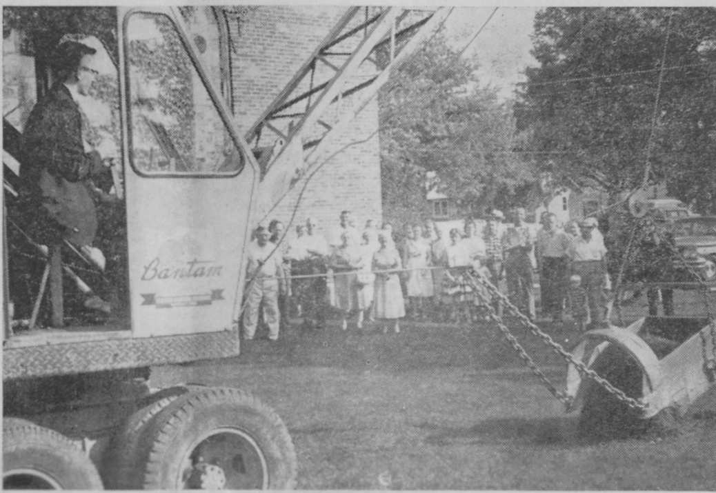
GROUND BREAKING ceremonies for the new school last fall saw the Rev. Walter C. Pieper, pastor, at the controls of this dragline. Members of the congregation watch the ceremony in the background. The building was completed during the winter.
