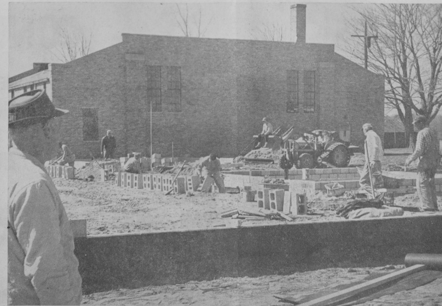
PROGRESS on the new Tawas City elementary unit is pictured above. O. S. Rose, general contractor, stands at left. Workmen are shown laying concrete blocks while the crew of Northern Plumbing and Heating makes an initial installation of pipe. Work is progressing rapidly during the favorable weather and
