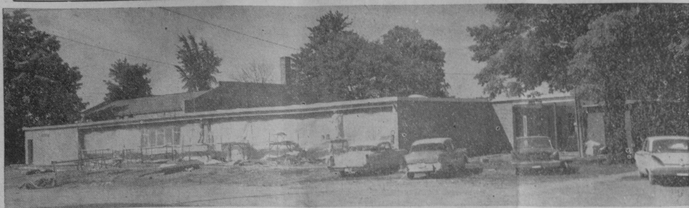
PROGRESS as of Tuesday morning on the new Tawas City elementary unit of Tawas Area Schools is pictured above. Plaster work on the building is now being completed. Work remaining includes laying of tile on floors and painting walls. School custodians will
