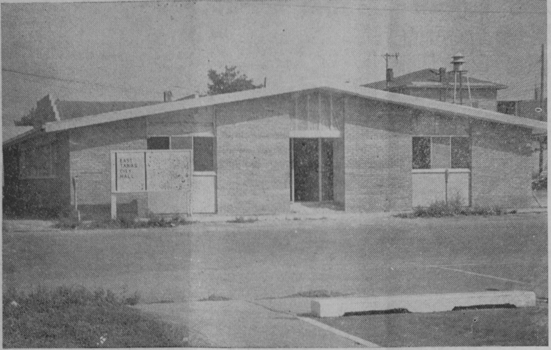
PROGRESS on the new city hall at East Tawas is pictured above. The building, located on the site of the old city hall, is to be completed this fall. It is of concrete block construction with brick veneer. General contractor is O. S. Rose Builders, Incorporated, Tawas City. Architect was Carl Schulwitz.—Tawas Herald Photo.
